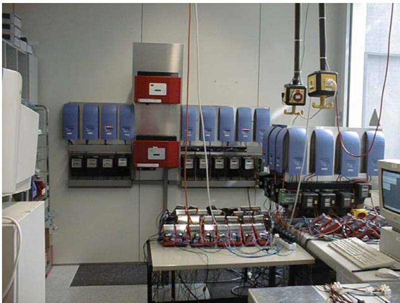
Fig. 4: Measuring- and Feed-in station
