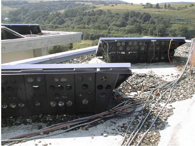
Fig. 7: test system is mounted on ventilated troughs
