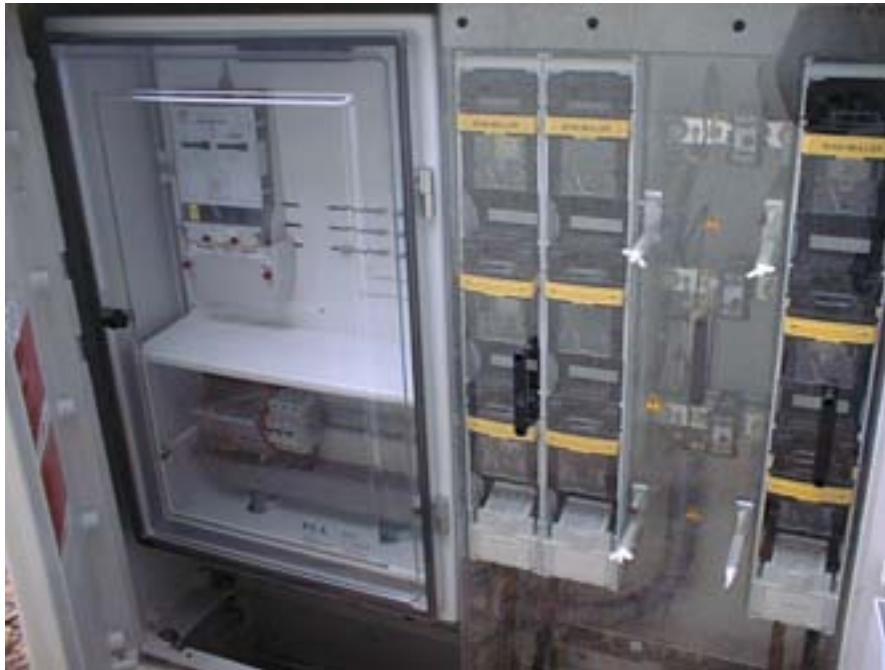
Abb. 23: Innenansicht des Messwandler-Schranks
